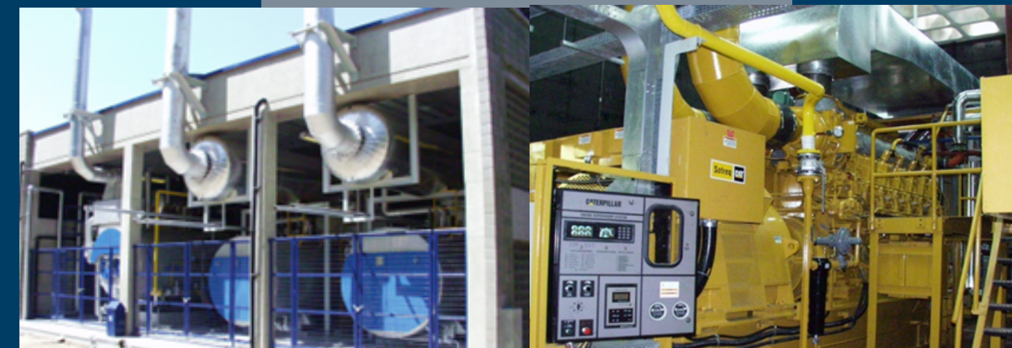
TWO HEAT RECOVERY BOILERS AND ONE STAND-BY BOILER
