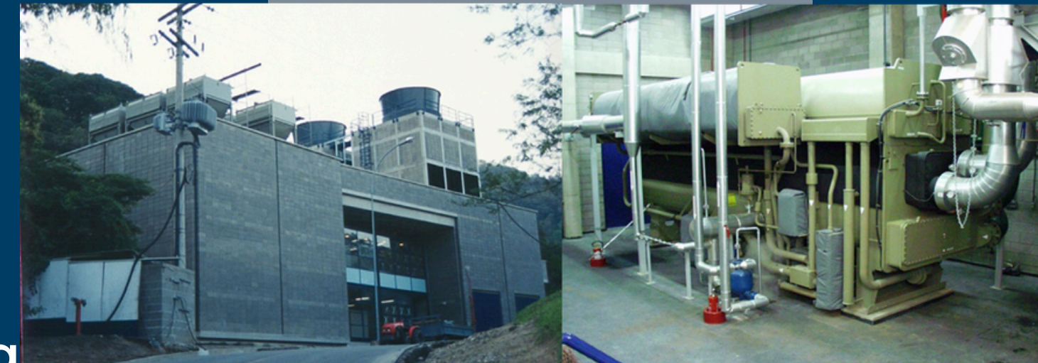
The Cogeneration Plant
